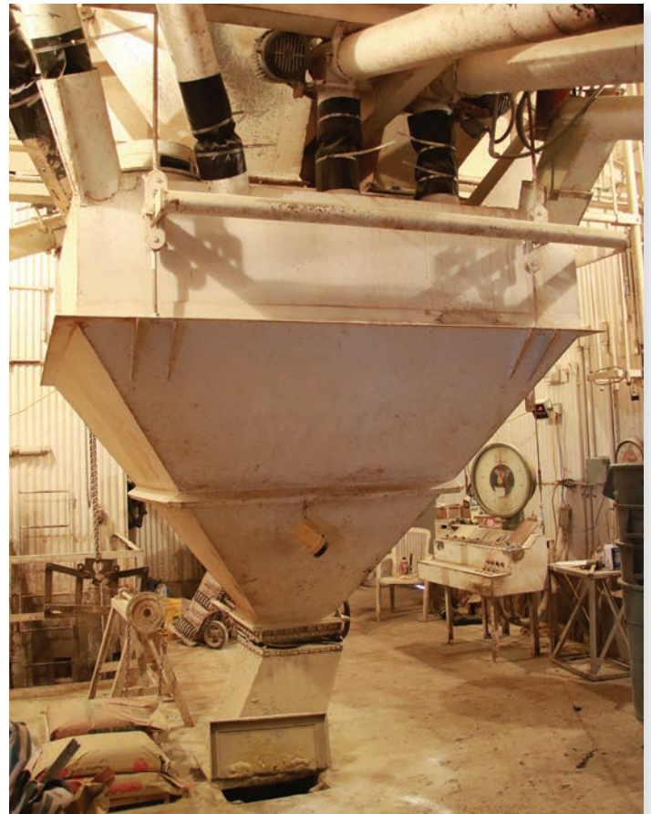
The main batch hopper inside the mill is used to mix the ingredients that make up the feed.
